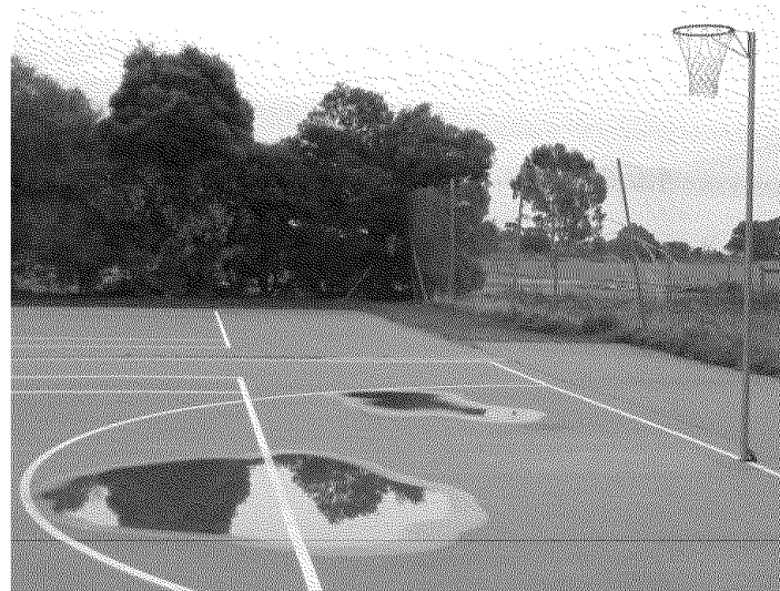
Figure 25: Netball courts showing water pooling, old fence and addition built onto courts to meet regulations
