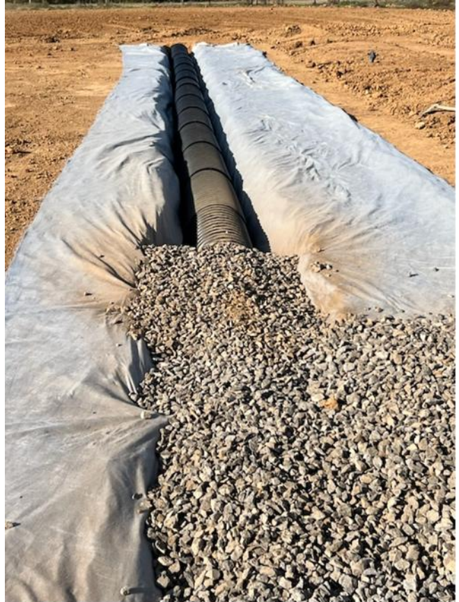
Image 18: Backfilling of Wick Trenches, with Geotextile fabric lining the trench before backfilling with suitable sized rock and arch drain.
