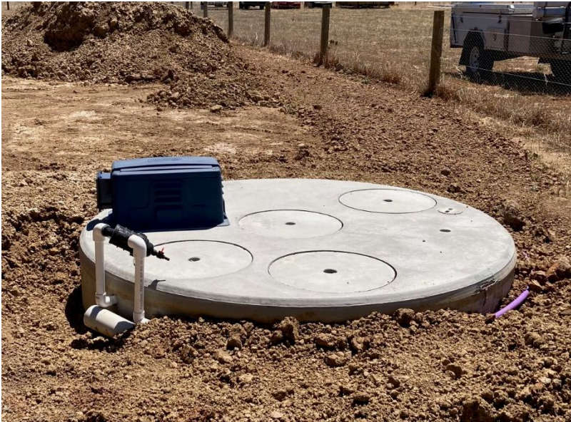
Image 10: Top of a packaged treatment plant – only the lid, control box and filter visible once backfilled
