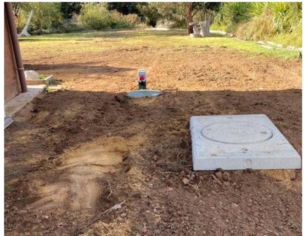
Image 9: Only the lid of the septic tank and pumpwell with alarm are visible when backfilled.
